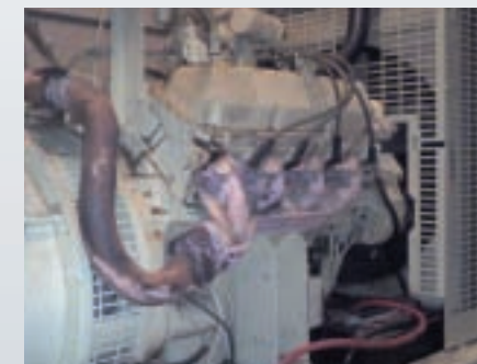
Visual Image of Generator
