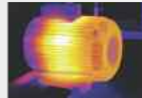
Motor: Internal Winding Problem
