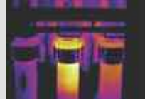
Electrical: Hot Fuses
